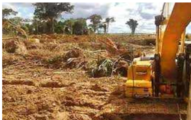
Image showing heavy tractor leveling a place as a follow up to deforestation Source: forestpeoples.org
